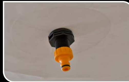
Central Drainage Point
